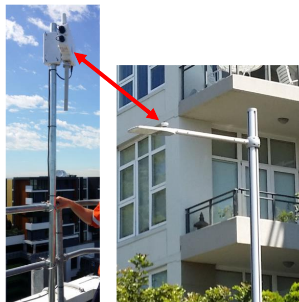
Pic1: Two-way wireless communication between WAP (on-left) and RF Node attached on LED Luminaire located at 2.5 km from WAP
